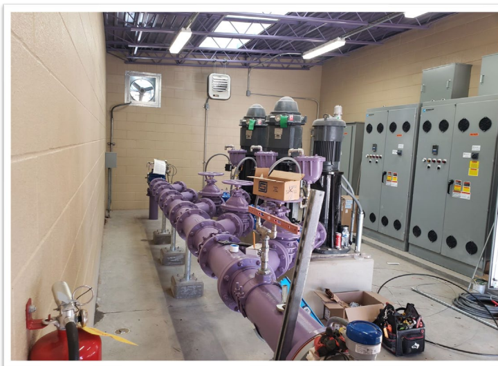
Non-potable system photo - Overlook booster station
