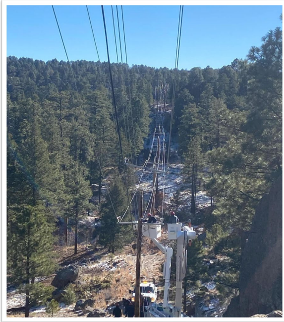
Electric linemen work to repair power lines damaged by trees that fell in a morning windstorm.
