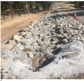
Erosion control on a drainage channel
