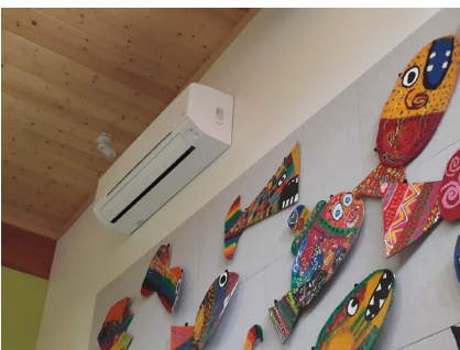
Nature Center HCAC Unit Installed
