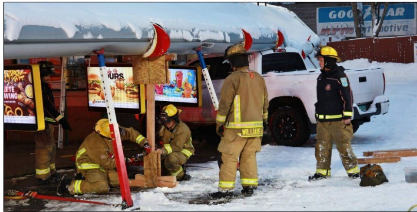
Crews respond to a structure collapse of the Sonic awning due to heavy snow
