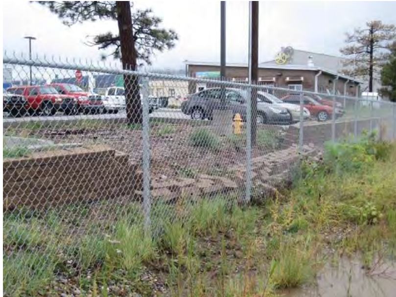
Figure 4.31. Damage to Retaining Wall at ECO Station
