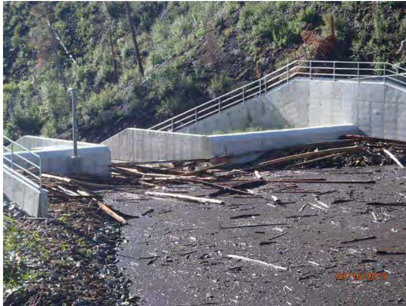
Figure 4.33. Debris at Los Alamos Reservoir Spillway
