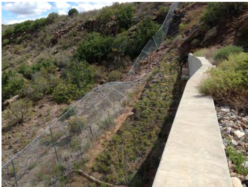
Figure 4.32. Debris/Fence Damage at Airport
