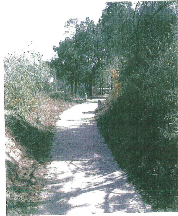
Need erosion control
