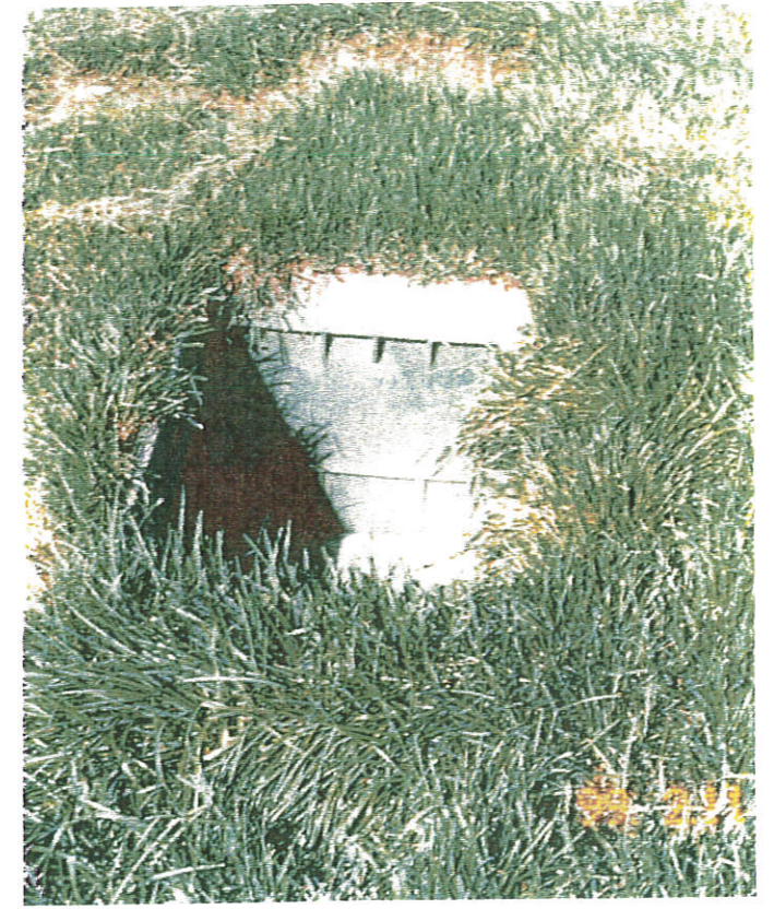
Repair/replace valve box
