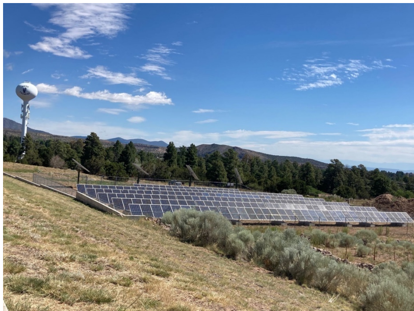
Solar array on North Mesa near Middle School
