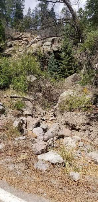
Path down the canyon wall the water took to form the pond.
