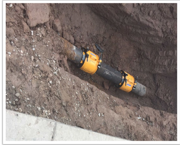
Water Distribution System photos - 33rd Street Pipeline Break/Repair (Aspen School Area) Crews cut out broken pipe segment show in the left photo, and repaired with new ductile iron pipe piece and two repair couplings (right photo).
