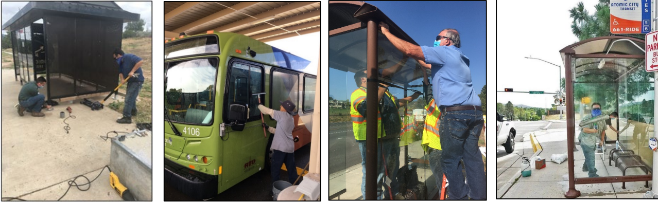
Employees clean and disinfect buses and bus shelters and perform bus stop maintenance
