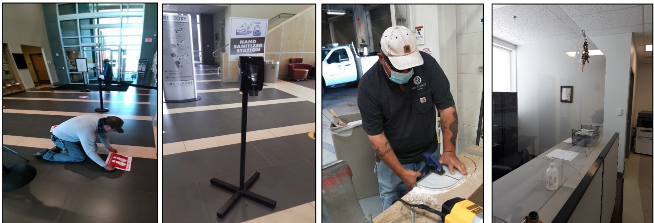
Crews installed floor decals and fabricated hand sanitizer stations and protective barriers at County buildings
