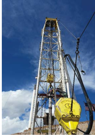
Drilling of the Otowi well 2 in Los Alamos Canyon. This coming year, construction will begin on the well house and installation of the pumping equipment.
