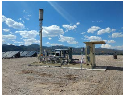
Landfill Gas Extraction System
