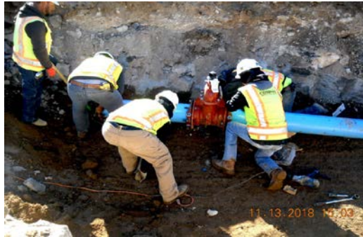
Construction crews install a waterline at the El Mirador subdivision in White Rock.
