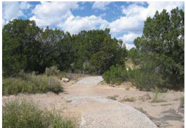
Continue to monitor the condition of the low-water crossing
