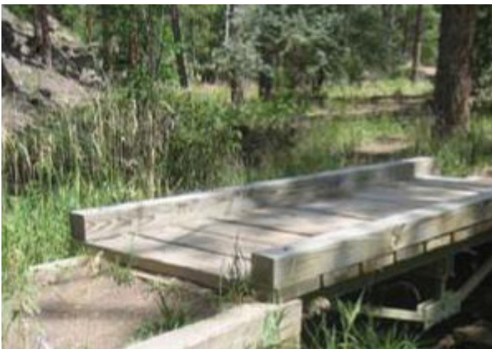
Monitor bridge condition.
