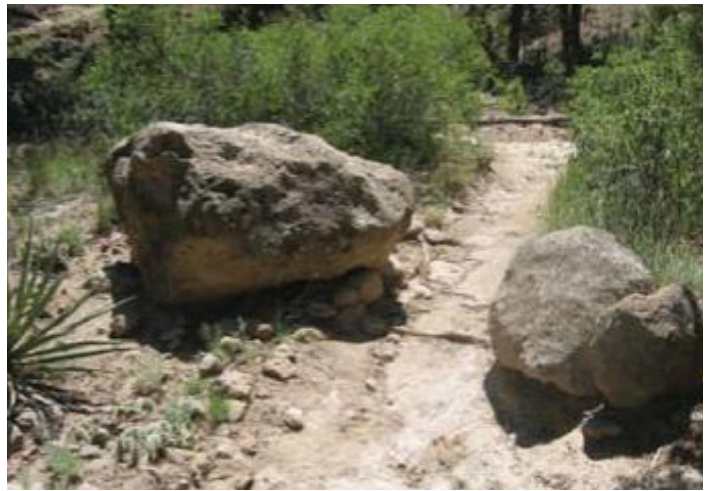
Repair erosion damage at the foot of the stairs.
