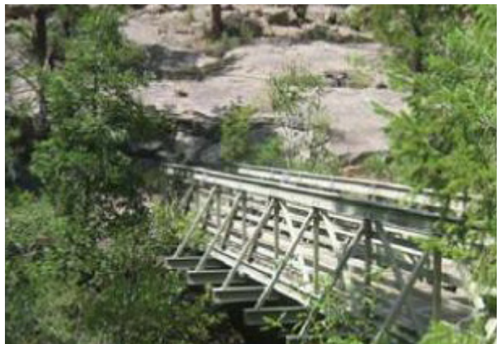
Monitor bridge condition.
