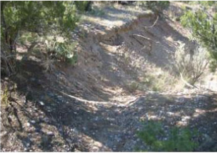
Reroute short eroded section just south of the badlands.
