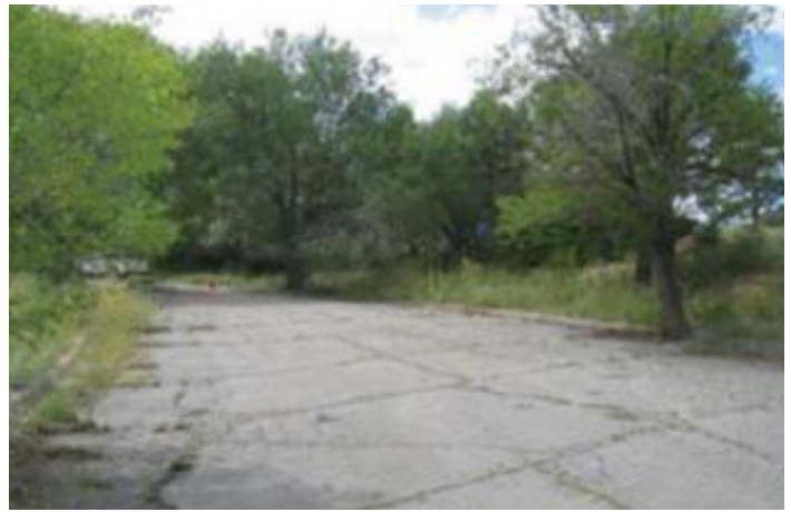
Establish improved parking at trailhead and install mini-kiosk and repair damage from street runoff to the trail.
